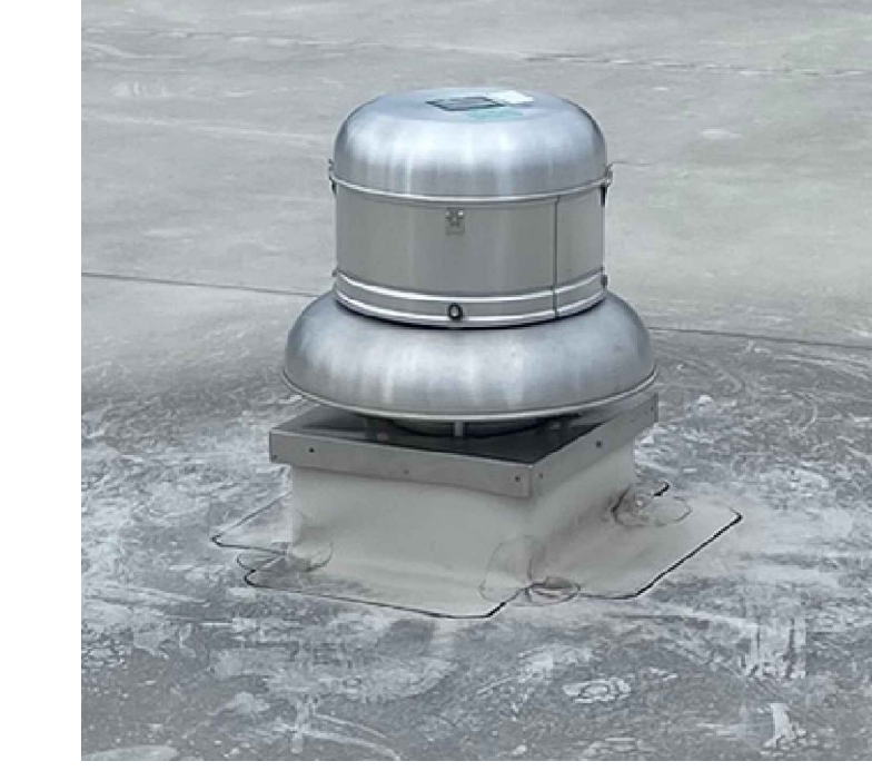
TYPICAL EXHAUST FAN CONDITION
