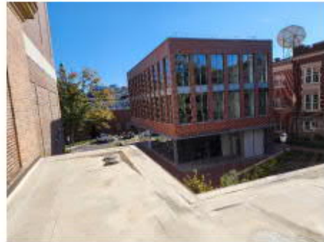
Photo #8 Low Roof between the Memorial Hall and the Curtis Media Building (Roof 6)
