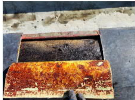
Photo #10 Asbestos-containing Black Material at the Parapet surrounding the Barrel Roof 1 (HA #14)
