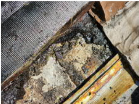
Photo #9 Asbestos-containing Black Tar Paper at the North Metal Roof A (HA #6)
