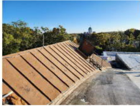
Photo #2 Metal Roof (Roof A) at the Barrel Roof north side (Roof 1)
