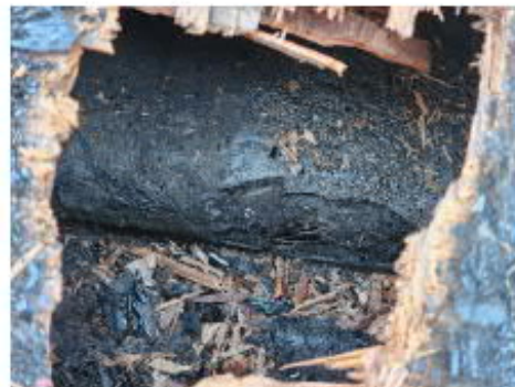
Photo #12 Asbestos-containing Black Tar Paper/Material underneath Plywood at the North Porte-Cochere Roof 5 (HA #24)
