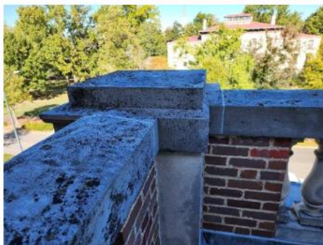
Photo #11 Asbestos-containing White Caulk on Balustrade at the North Porte-Cochere Roof Area 9
