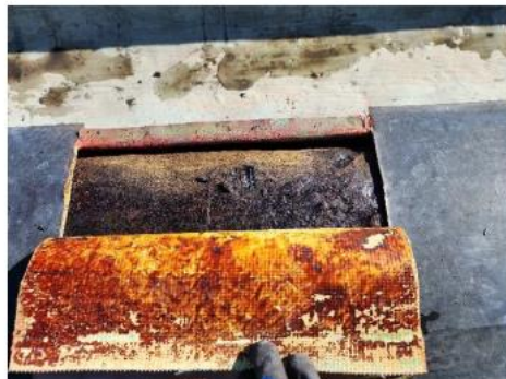
Photo #10 Asbestos-containing Black Material at the Parapet surrounding the Barrel Roof Area 1
