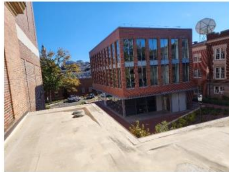
Photo #8 Low Roof between the Memorial Hall and the Curtis Media Building (Area 6)
