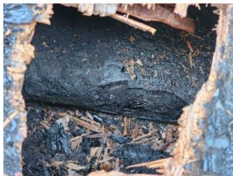
Photo #12 Asbestos-containing Black Tar Paper/Material underneath Plywood at the North Porte-Cochere Area 9
