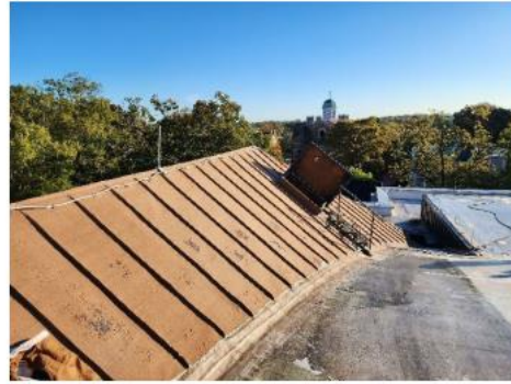
Photo #2 Metal Roof (Area A) at the Barrel Roof north side (Area 1)
