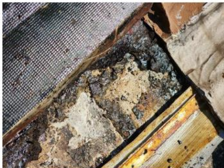
Photo #9 Asbestos-containing Black Tar Paper at the North Metal Roof Area A
