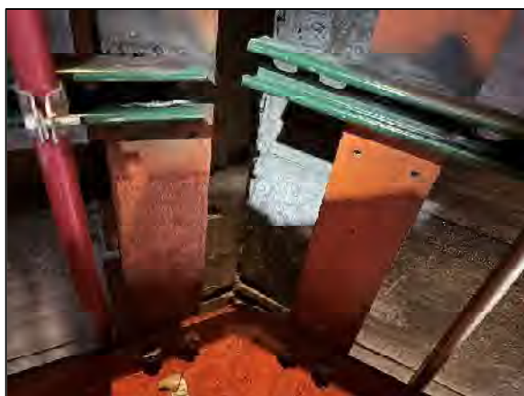
PHOTO 3 View of Sampling Location for BB-2 Central Wing - Attic 2% Chrysotile
