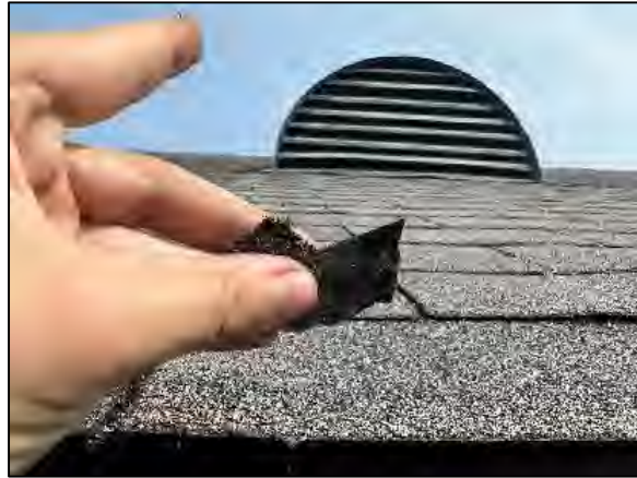
PHOTO 8 Close-up view of Sample BB-4 South Wing of Original Building – South Perimeter (NONE DETECTED)
