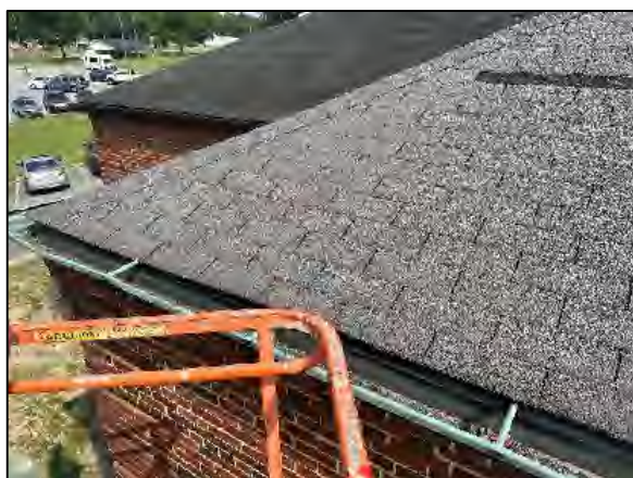
PHOTO 7 View of Sampling Location BB-4 North Wing of Original Building – South Perimeter (NONE DETECTED)
