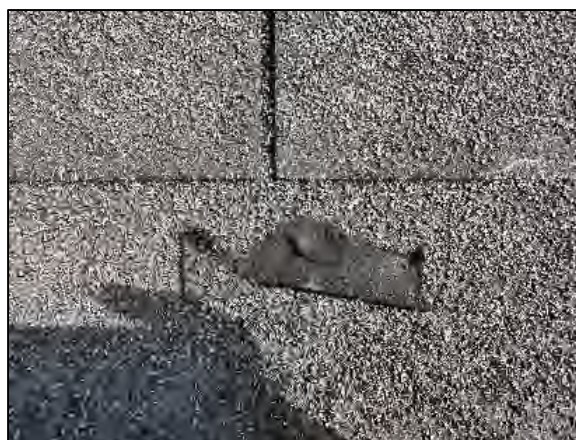
PHOTO 8 Close-up view of Sample BB-4 North Wing of Original Building – South Perimeter (NONE DETECTED)
