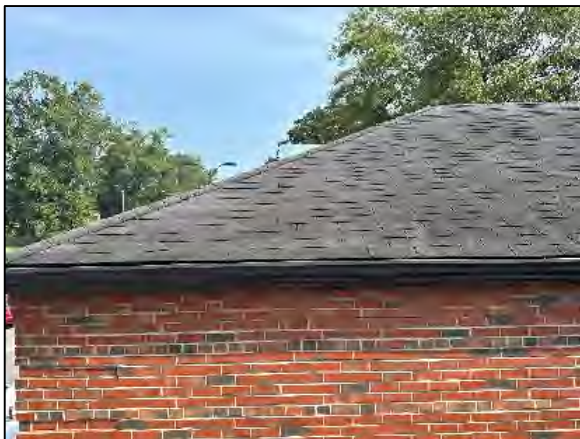
PHOTO 11 View of Sampling Location BB-6 Northwest Mechanical Room Addition – South Perimeter (NONE DETECTED)
