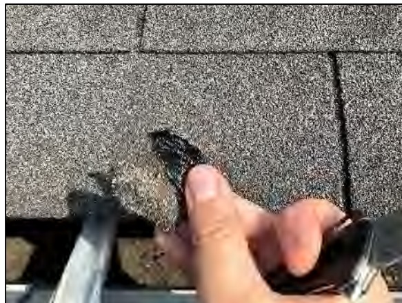
PHOTO 12 Close-up view of Sample BB-6 Northwest Mechanical Room Addition – South Perimeter (NONE DETECTED)
