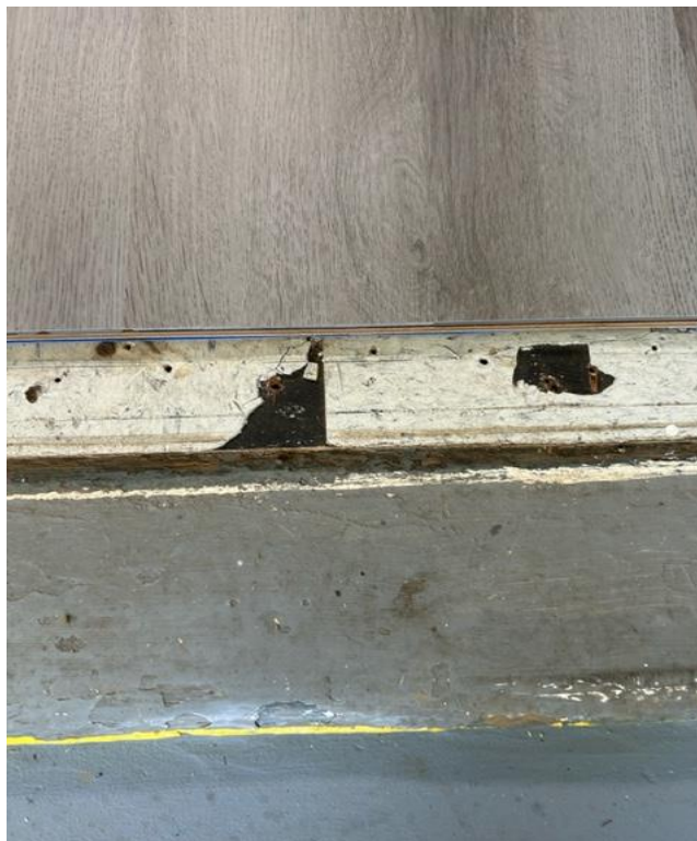
Typical of Asbestos-Containing Floor Tile Mastic located beneath finish flooring.
