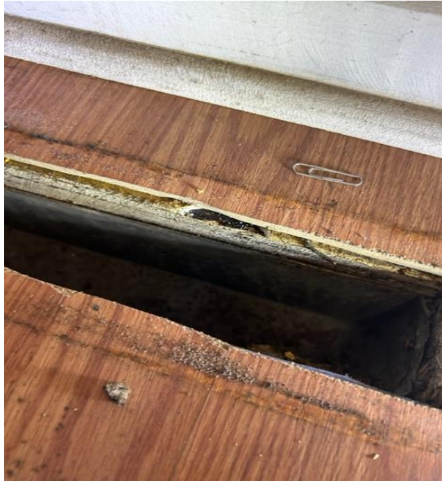
Typical of Asbestos-Containing Floor Tile Mastic located beneath wood flooring
